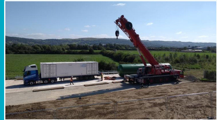
SMR and Bullet move from Kiwa House to the new SMR site. A reinforced crane base was laid to take the weight of the bullet move.
