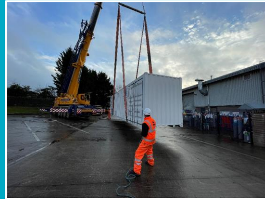
SMR delivery to Kiwa House for safe storage whilst the groundworks take place on site
