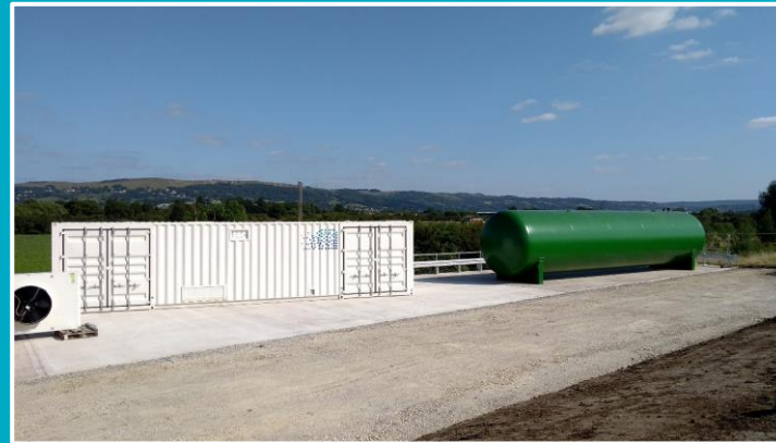
SMR Installed an in location
